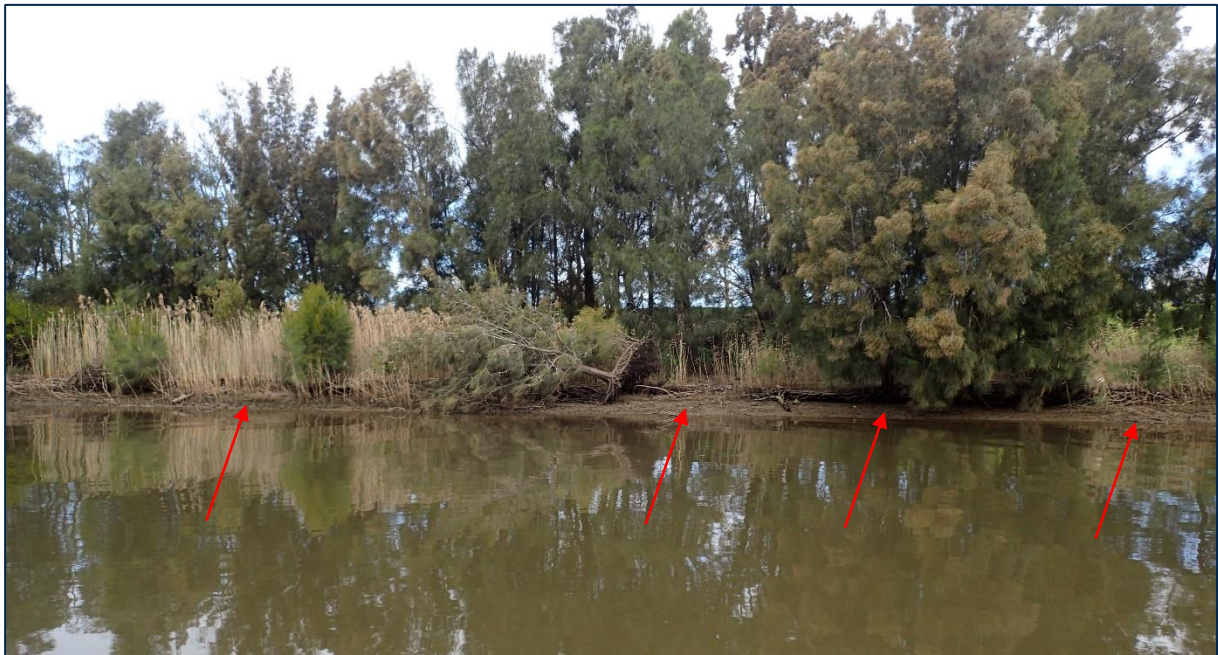
Figure 6: Representative photograph of bank scour along a bank section with an existing tidal bench. Note the partially detached tree and root mat in centre of picture and adjacent bank scour (identified by red arrows). Location is 990 m upstream of the Terara Sands depot site. Flow is right to left.
