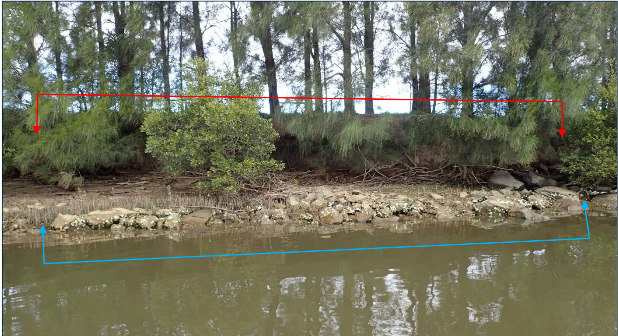
Figure 2: Representative photograph of bank scour along a bank section (identified by red arrows). Blue arrows identify a length of disarticulated bank protection stonework. Note the tidal bench accretion on the lee (downstream) side of the stonework. Flow is right to left. Bank height is about 1.5 m. Location is 1,060 m downstream of Terara Sands depot site.
