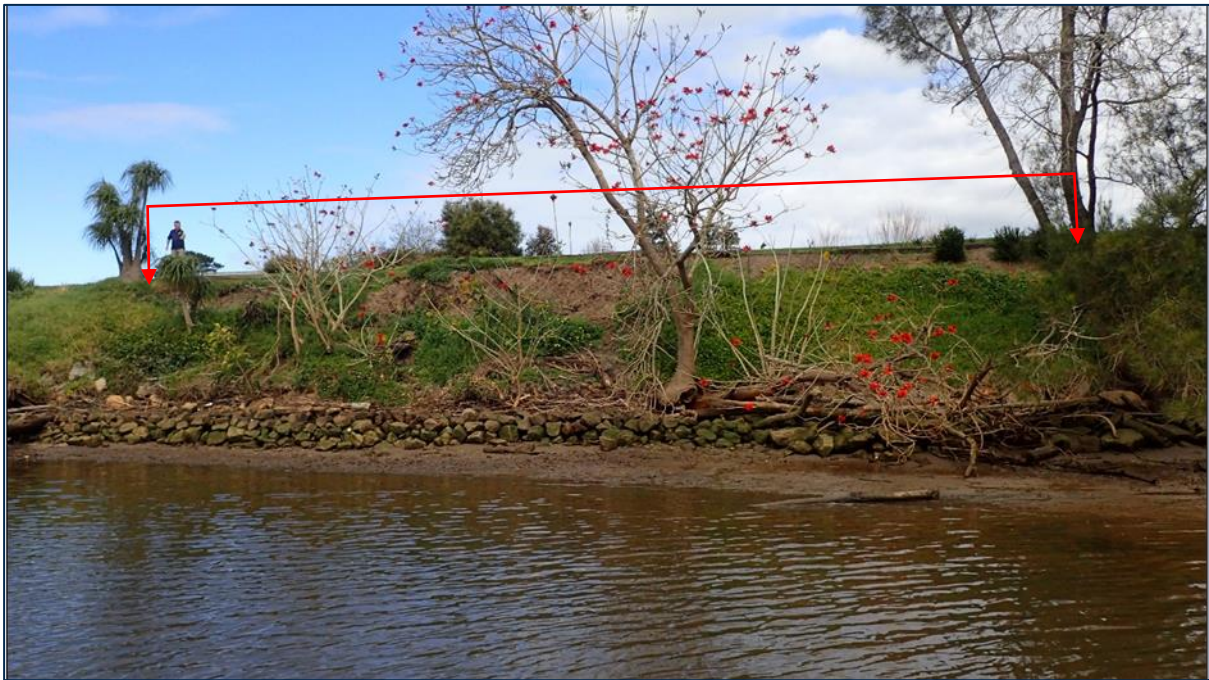
Figure 1: Photograph of slumped bank and levee section documented in Council's RFI, located approximately 50 m downstream of the Terara Sand depot site.
